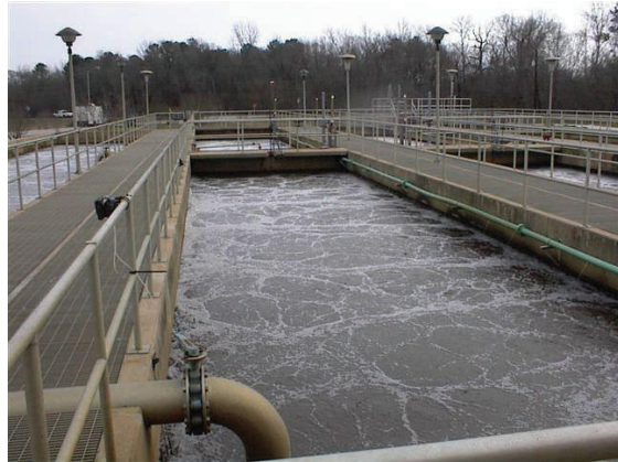
Wastewater Treatment Plant Aeration Basin
